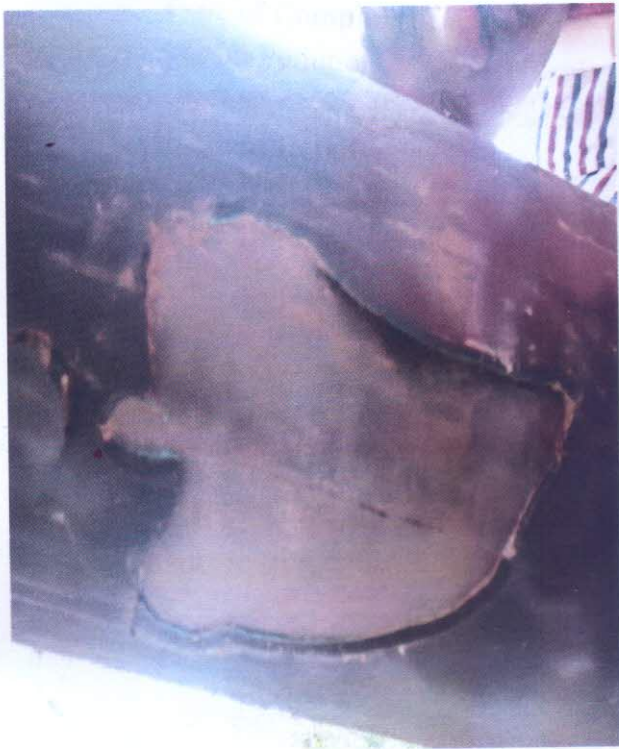
SPILL POINT AFTER EXCAVATION
